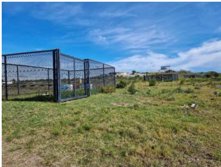
Domestic Water Supply Production Boreholes within the Jeffrey's Bay Wellfield
